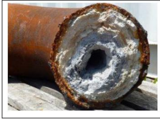
Gambar 2. Silica scaling di Dieng geothermal plant (Rahman et al. , 2023).
